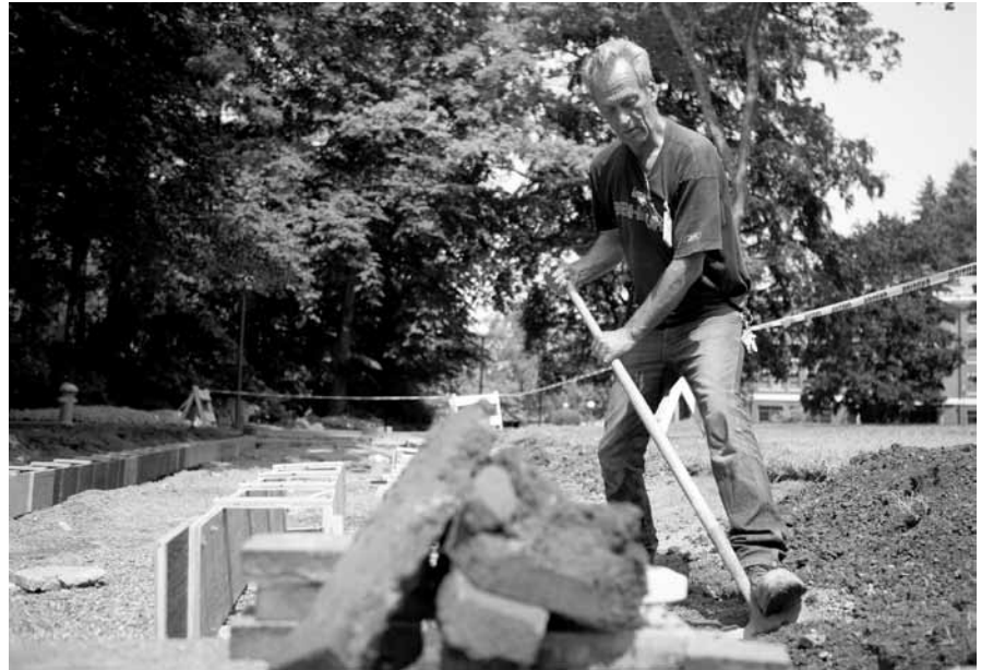
Denny Bouma, a maintenance mechanic with WWU Facilities Management, digs out space for a concrete footing under one of the brick walkways under repair in front of Old Main.
